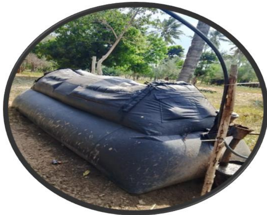
Figure 2: Small scale- Home-based biogas unit
